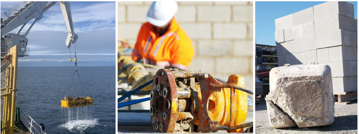
Left to right: Recovery of debris. Dismantling recovered hydraulic flying leads. Recycling concrete mattress blocks into building blocks.
